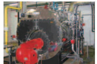
A boiler at SNR that was converted to run on natural gas
